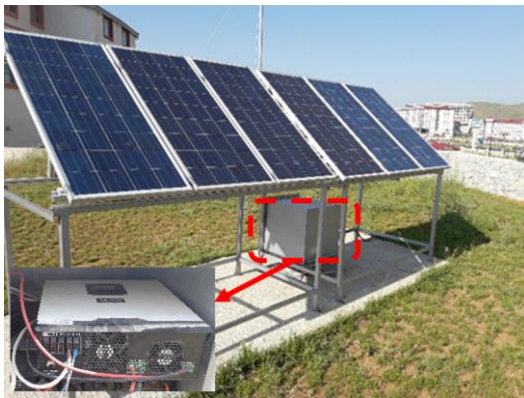
Fig. 2. PV panel and inverter
