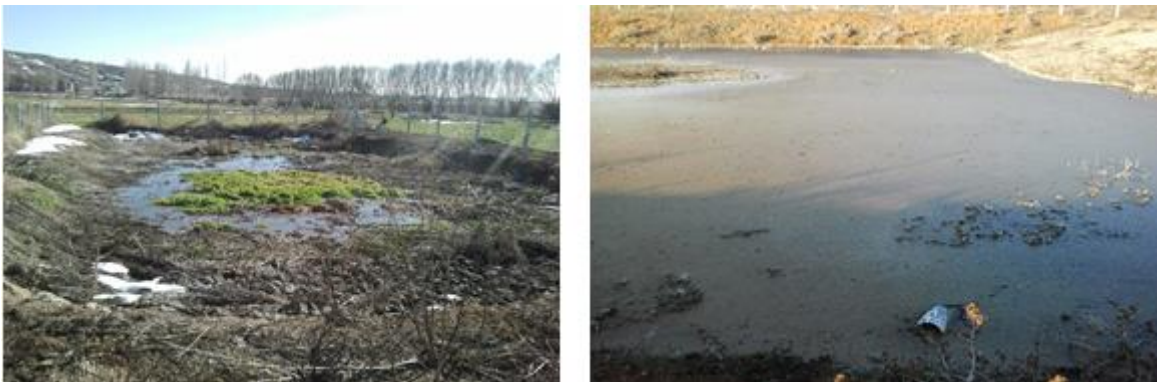
Figure 6. Clogging due to unsuitable media
