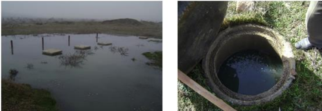
Figure 7. Clogging septic tank
