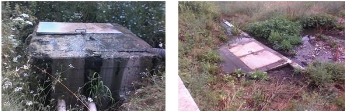
Figure 5. Clogging due to use unsuitable inlet and outlet structures
