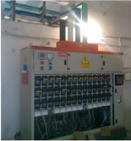
Figure 3. Transformer center from inside -2 (control room)
