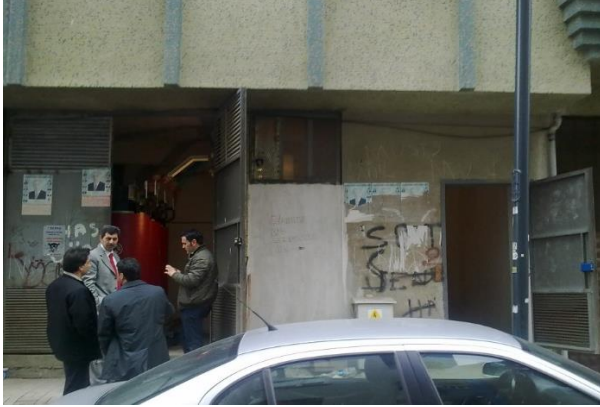
Figure 1. The transformer center from outside
