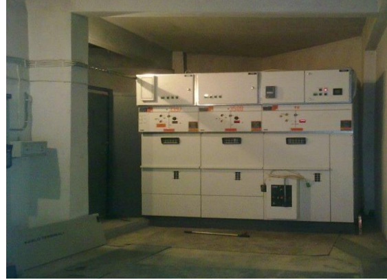
Figure 2. Transformer center from inside -1 (control room)
