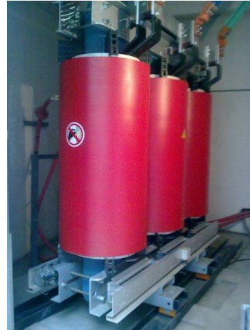
Figure 4. Transformer center from inside -3 (transformer room)
