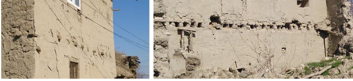
Figure 5. Photos that show the top floor tile
