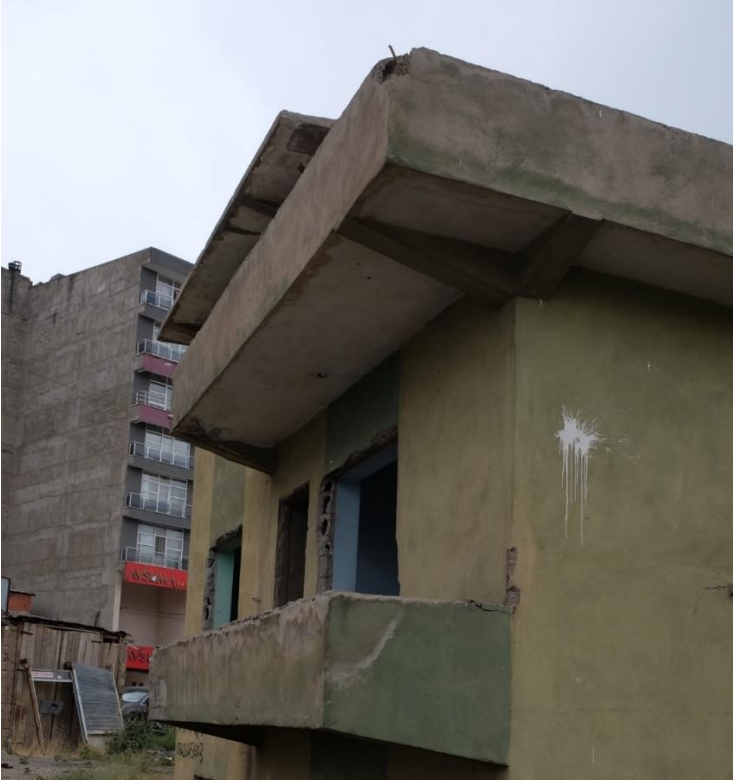
Figure 7: Damaged building at the city center (Photo by the author, August, 2017)
