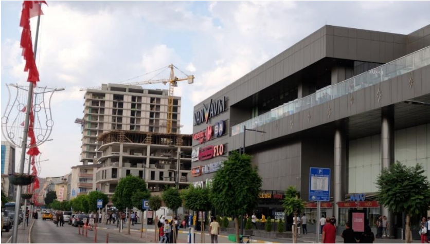
Figure 6: High-rise buildings under construction beside a new shopping mall (Photo by the author, August 2017)
