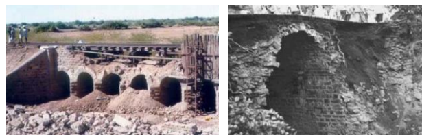
Figure 2. Bridges damaged by the 2001 Bhurj earthquake and the Koyna earthquake in India
