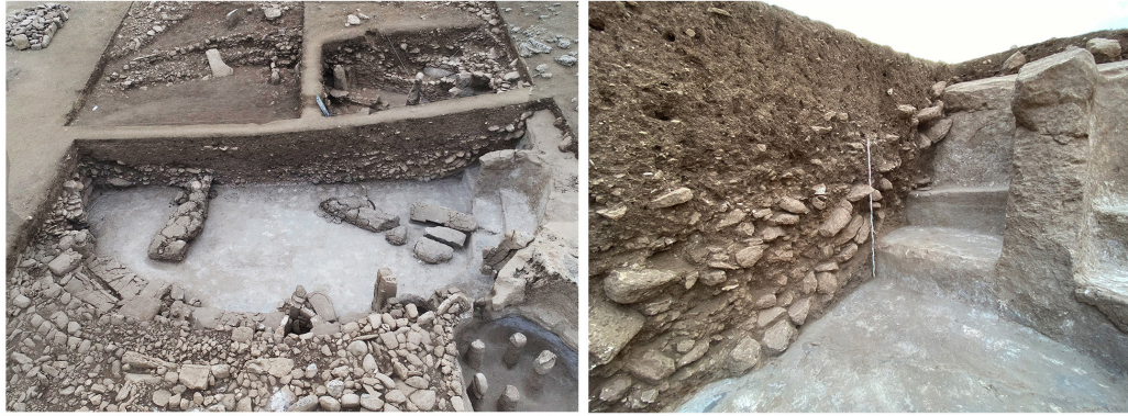
Fig. 4. Photographs of the section in Str. AD showing the demolition process of the building from the periphery towards the center.
