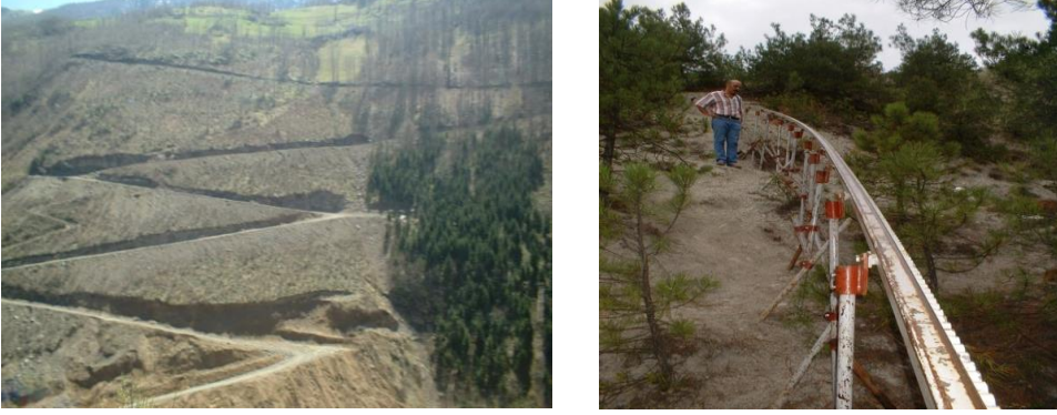
Şekil 5. Tekray sisteminin dik arazide kurulumu Figure 5. The installation of the Tekray system on steep terrain
