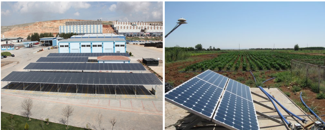
Figure 11. Gaziantep Water and Sewerage Administration (GASKİ) General Directorate Solar Car Park and Solar-Powered Drip Irrigation System [21]
