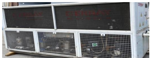
Fig. 5 Cooling system with two-compressor
