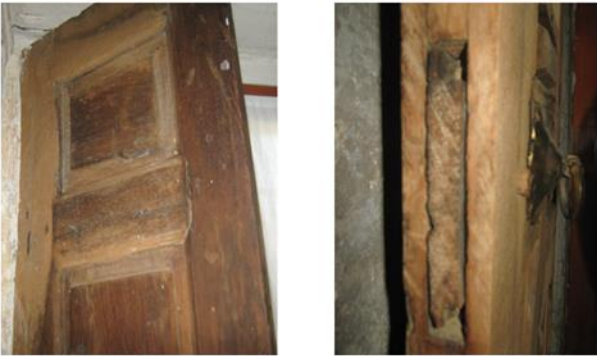
Figure 11. Corrosions seen in window shutters.
