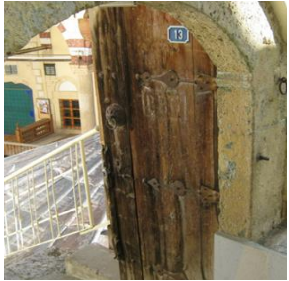
Figure 8. Corrosion seen in metal parts of the outer courtyard door and the rotting of wood.
