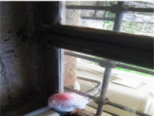
Figure 12. Ac Pipes going through the window frame.
