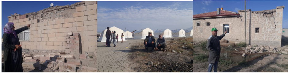
Figure 3: Examples of material damages after 21.09.2020 Niğde, Bor Earthquake (Anadolu Ajansı, 2020)
