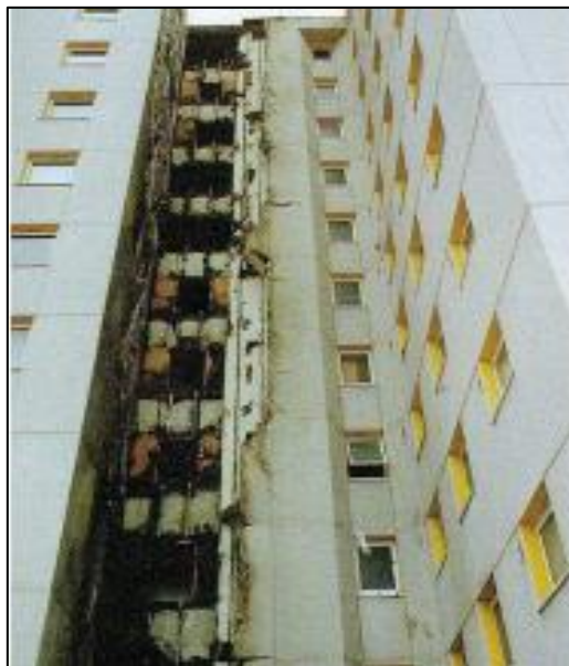
Figure 3. Chimney effect and fire spread due to façade movement [15]
