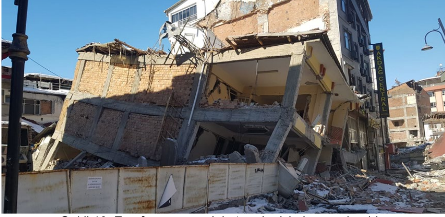
Şekil 10: Zayıf ve yumuşak kat nedeniyle hasar alan bina Figure 10: Building damaged due to weak and soft storey
