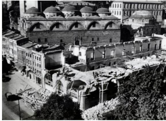
Fig. 6. Demolishment of Tophana Barracks Located In Front of Tophana-i Amire, During the Opening of Kemeraltı Street. 16
