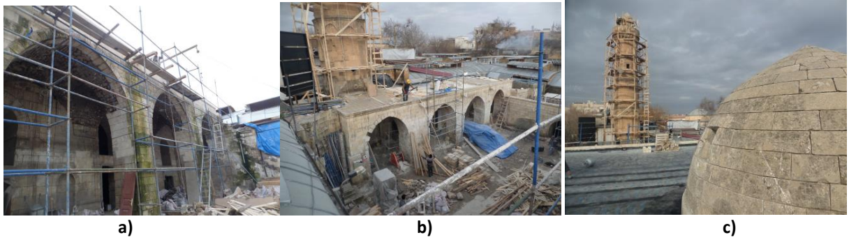
Figure 12. a) The removal of the additions to the portal b) The removal of the added stories onto the North side c) Cleaning in the minaret (Şanlıurfa Regional Board for the Conservation of Cultural and Natural Heritage and Şanlıurfa Regional Directorate for Foundations Archive, 2017).
