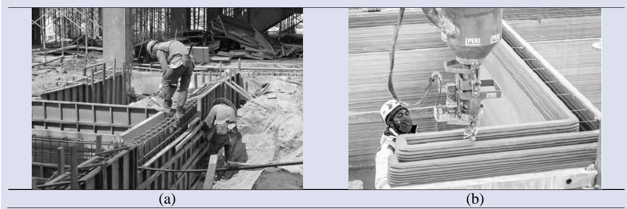
Resim 9. (a) Geleneksel betonarme sistem bina inşası ve (b) 3D Baskı ile bina üretimi Figure 9. (a) Traditional reinforced concrete system building construction and (b) building production with 3D Printing
