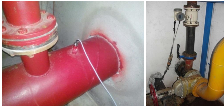
Figure 5. Temperature measurement at the inlet of the transmission pipeline (left), flow rate measurement at the outlet of the transmission pipeline (right).
