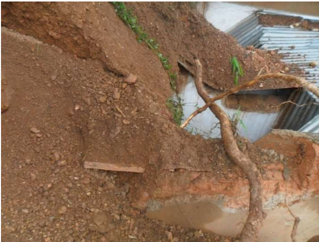
Fig.2 A house destroyed by a LANDSLIDE in North of Rwanda, a family of 6 people killed MIDIMAR, 2011
