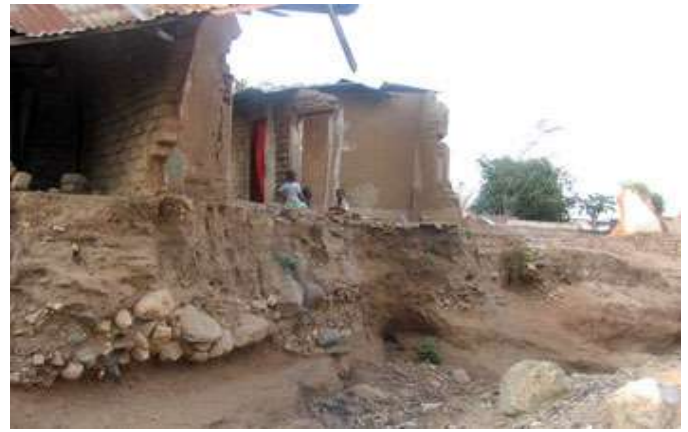
Fig.3 A house destroyed by lateral landslides
