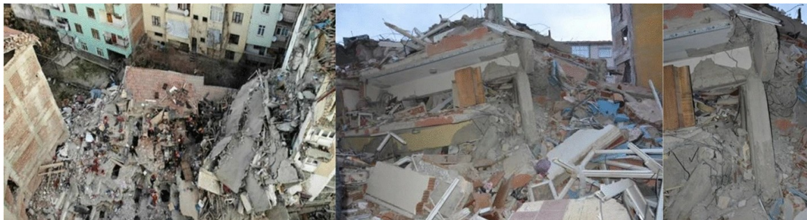
Figure 9: A view of the fully collapsed Aykent Building. URL 3: (Dogan et al., 2021)
