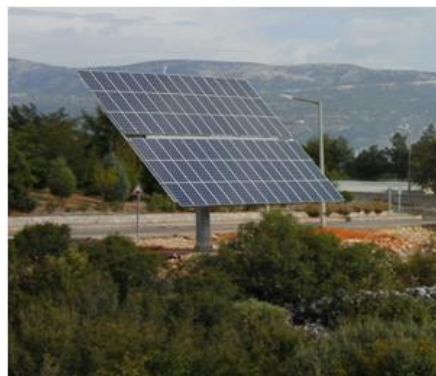
Figure 6: PV array at Mugla Sıtkı Koçman University campus (Eke and Senturk, 2012).
