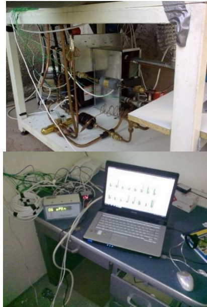
Figure 2. General view of the experimental setup used for space heating applications in GSHP
