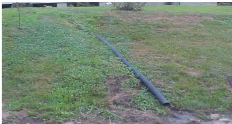
Figure 2. A typical straight pipe discharge (EPA Region 4, 2002).
