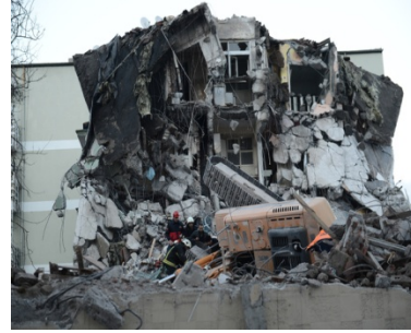
b) Demolition accident in Malatya
