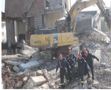
(a) Demolition accident in Denizli
